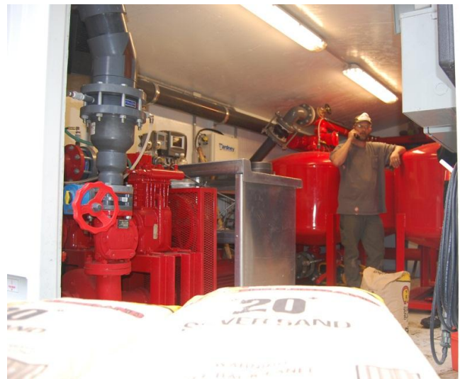
Chitosan mobile treatment equipment
